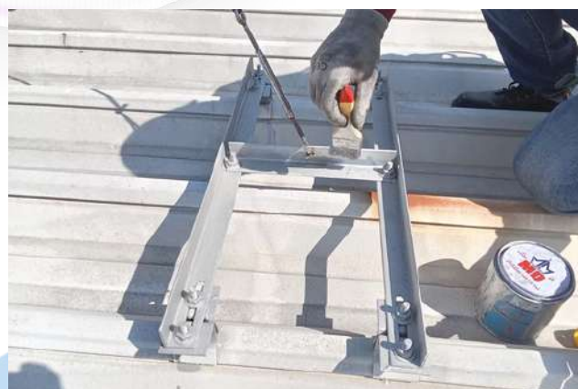
Lightning protection's support painting
