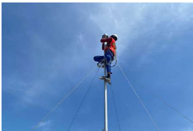
Head lightning protection remove for clean
