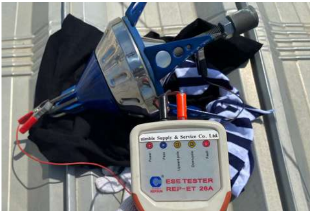
Head lightning protection testing
